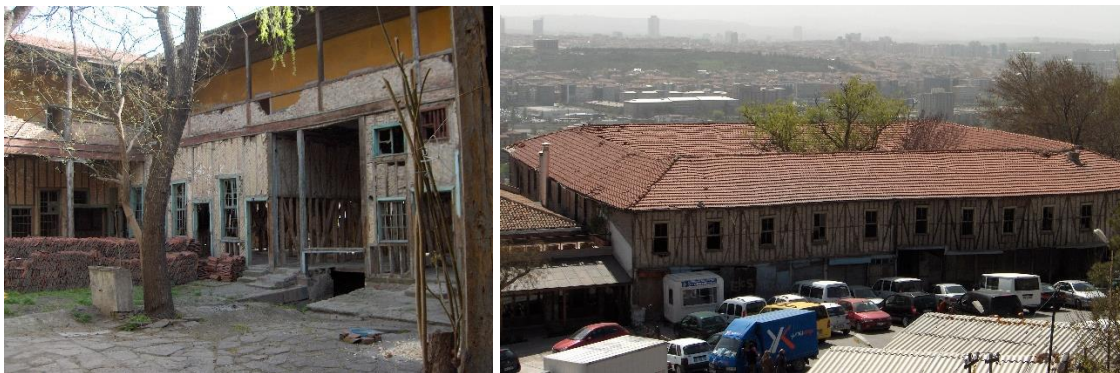
Figure 5. Çukurhan courtyard and exterior before restoration (Archive of Ankara Regional Directorate of Foundations)
