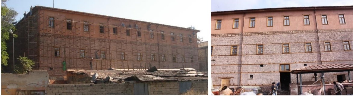
Figure 12. Spilled joints have been completed (Archive of Ankara Regional Directorate of Foundations)
