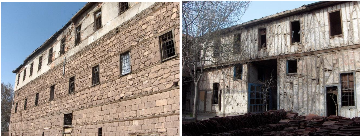
Figure 2. Çukurhan rubble stone and wood carcass system (Archive of Ankara Regional Directorate of Foundations)
